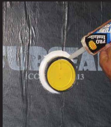
Applying sealant at all pipe terminations is an excellent way to complete a proper waterproofing job.
